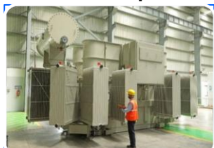
Oil Filled Reactors
